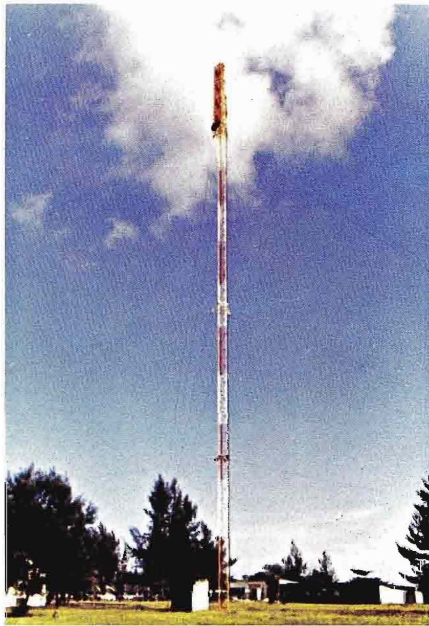
Antenna mast with microwave "Dish" for OB's.
